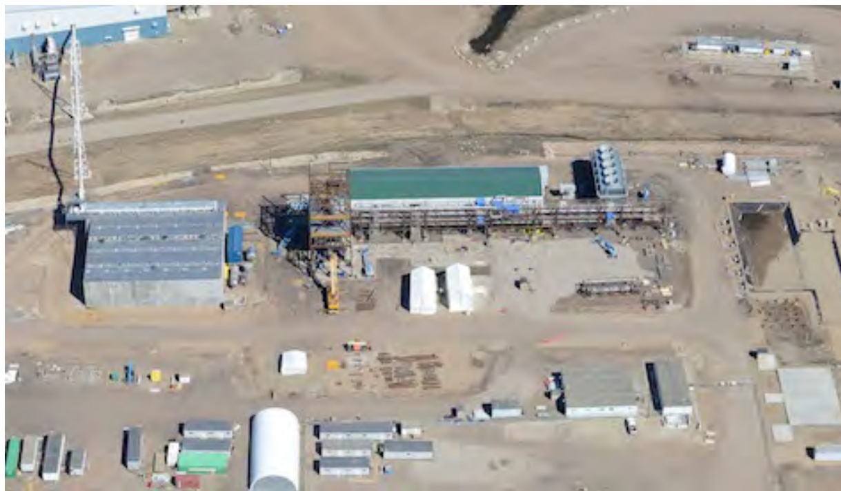
ENERKEM EDMONTON, ALBERTA, MSW GASIFICATION TO ETHANOL FACILITY UNDER CONSTRUCTION (PICTURE TAKEN MAY 2013), OPERATIONS EXPECTED IN 2013 (METHANOL)/2014(ETHANOL) (110,000 TPY PREPROCESSED MSW, 10 MILLION GAL/YR OF ETHANOL)
